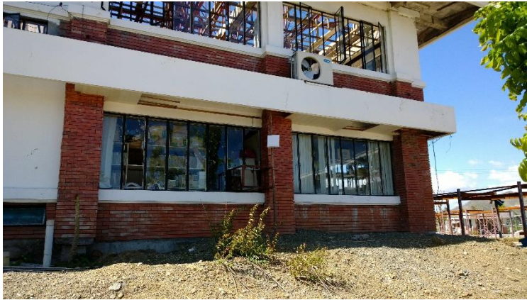
PSHS Administrative Building (the CPE antenna is the white square in the center of the photo).
